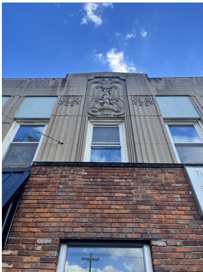
Figure 18. Primary (north) Façade, Frozen Fountain Detail, Hallie Wright
