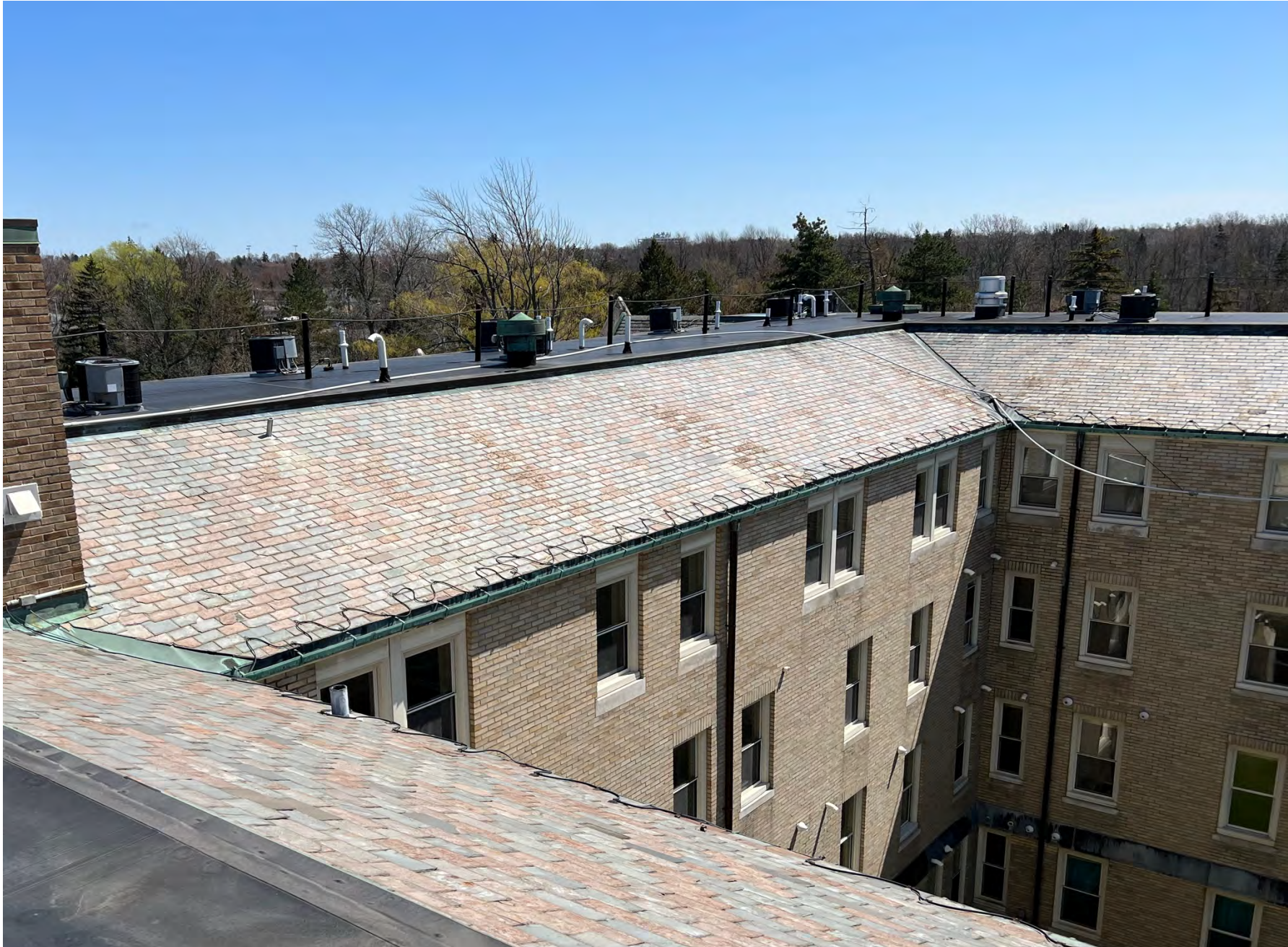
Photo of existing slate taken in May of 2022.
