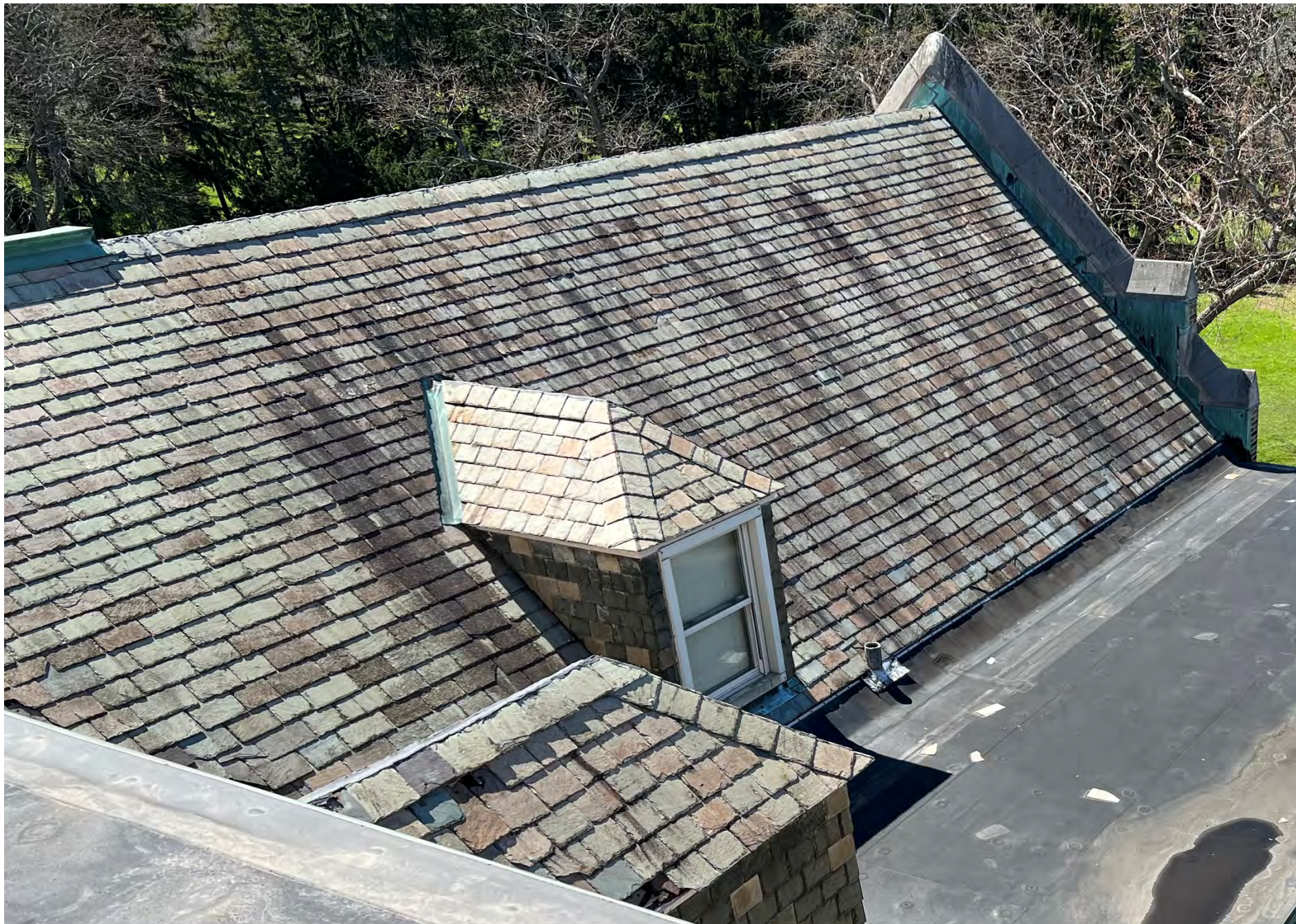
Photo of existing slate taken in May of 2022.
