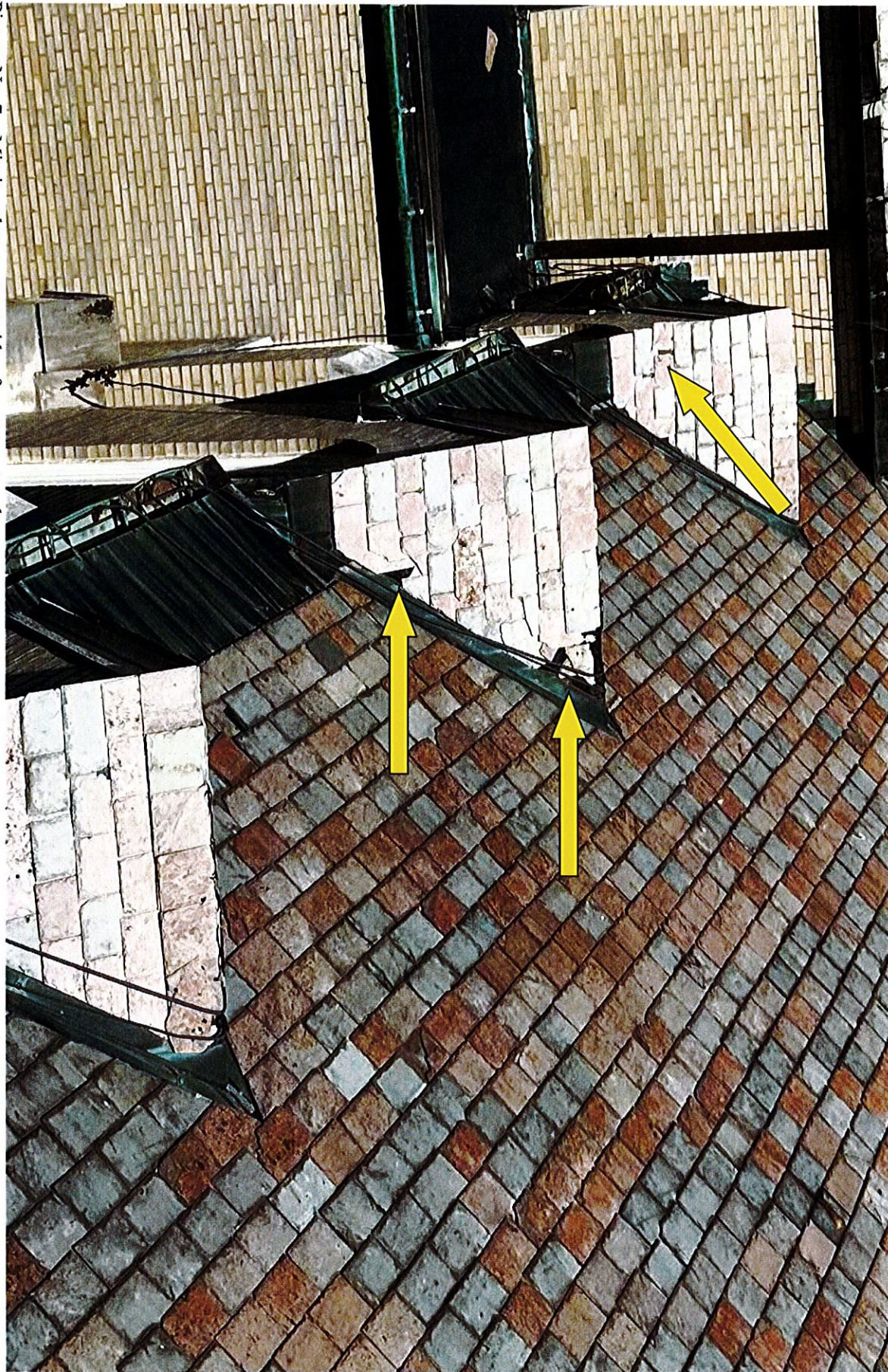
Picture No. 7 – Missing slate on west side of west courtyard.
