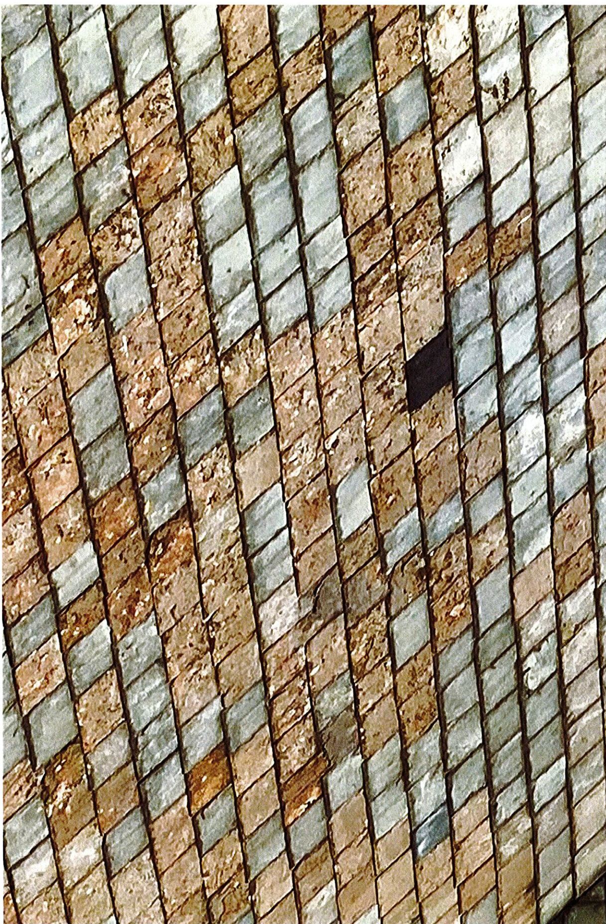
Picture No. 9 – Note how the slate is scaling and delaminating.
