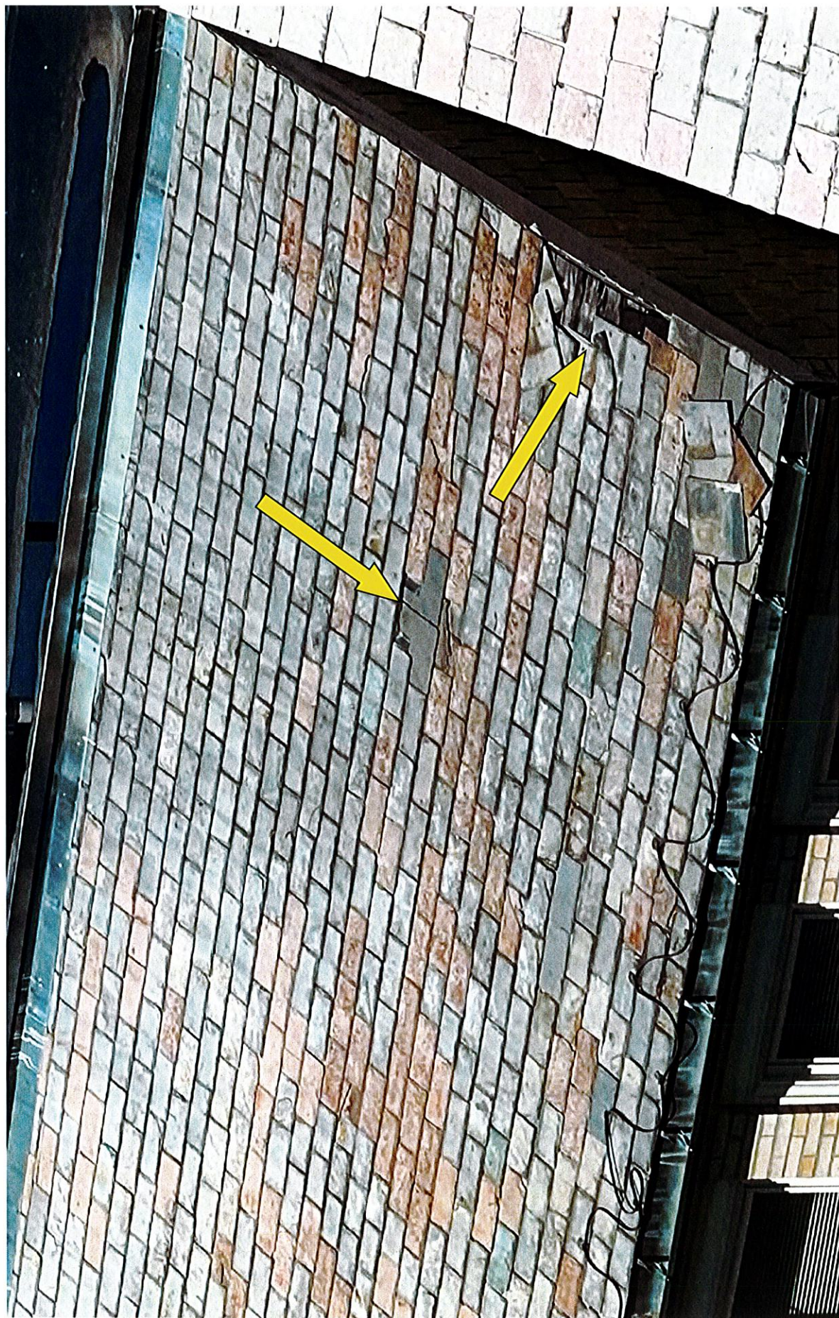
Picture No. 1 – Northwest corner of the west courtyard. Note the many missing slate, prior repairs, and scaling.
