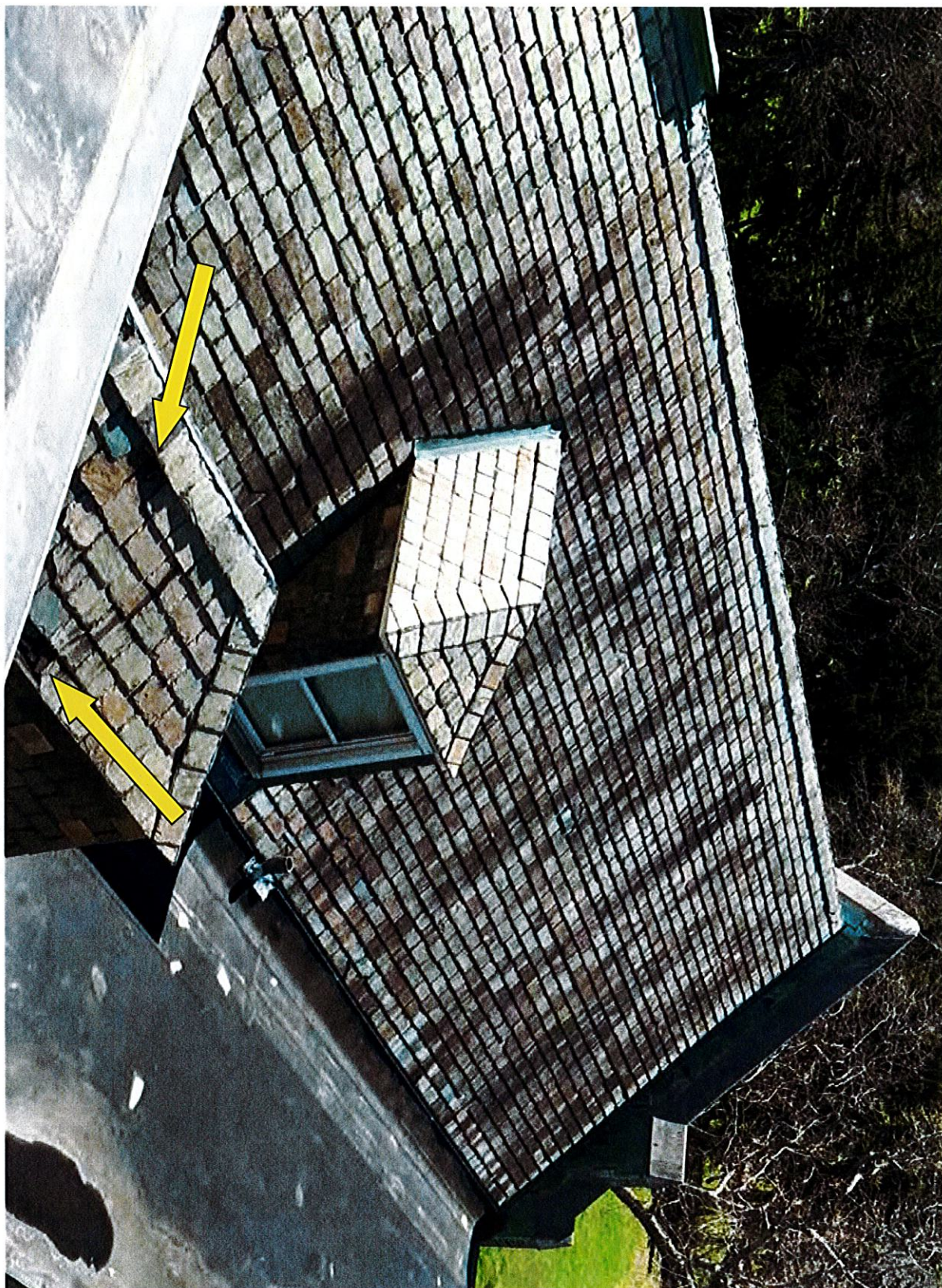
Picture No. 6 - Southwest corner of west elevation. Note the sealing, broken slate, and missing slate.
