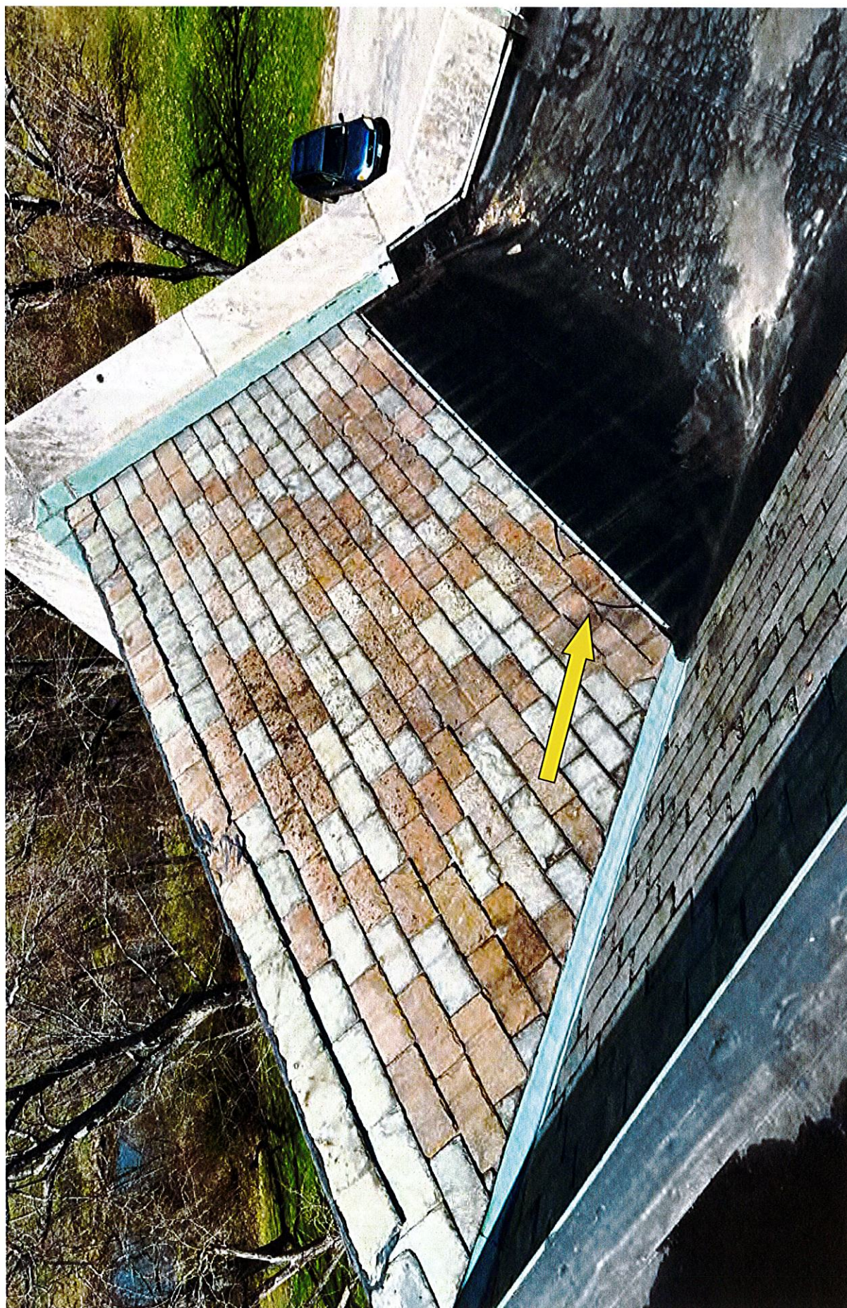
Picture No. 4 – Note the broken slate and the wide spread sealing on west side dormer roof.
