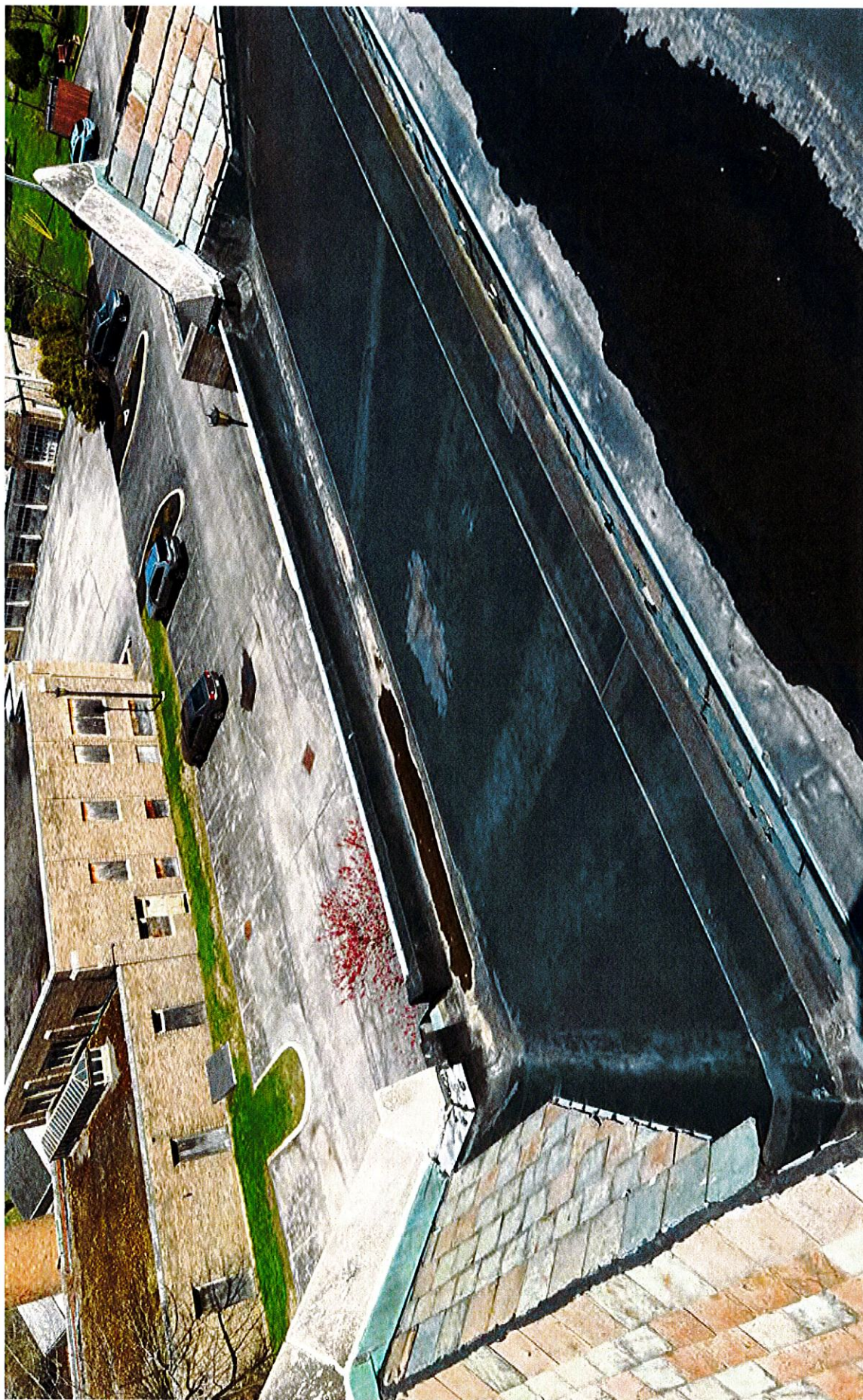
Picture No. 5 - Sloped/slate repair area on the west elevation has been covered with EPDM (rubber) membrane as a stop gap measure.
