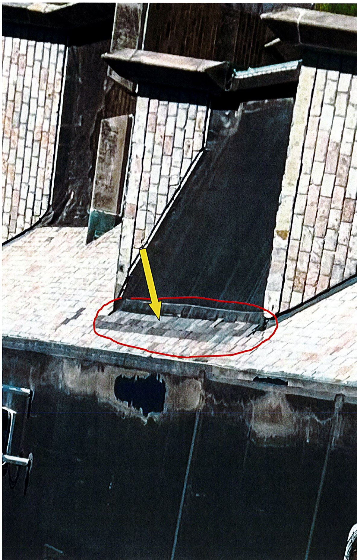
Picture No. 2 – Prior repair, south elevation, east side. Slate does not match.
